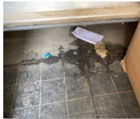
Photo 9. Floor was found soiled. Photographed 2-3-2026.
