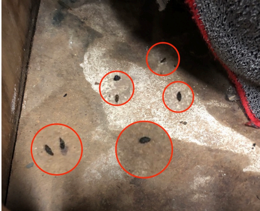
Photo 13. Examination room cabinet had vermin droppings (photographed on July 15, 2021).
