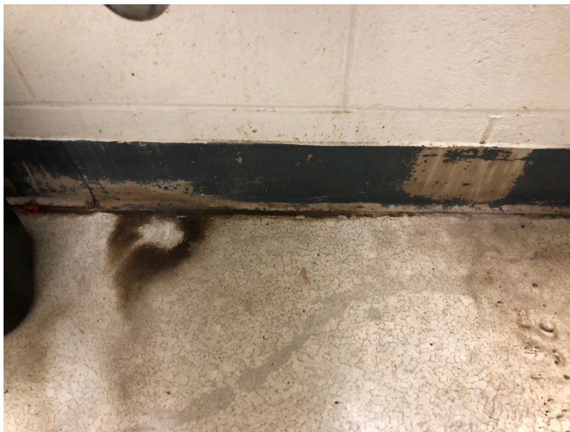
Photo 14. Unsanitary staff restroom (photographed on July 15, 2021).
