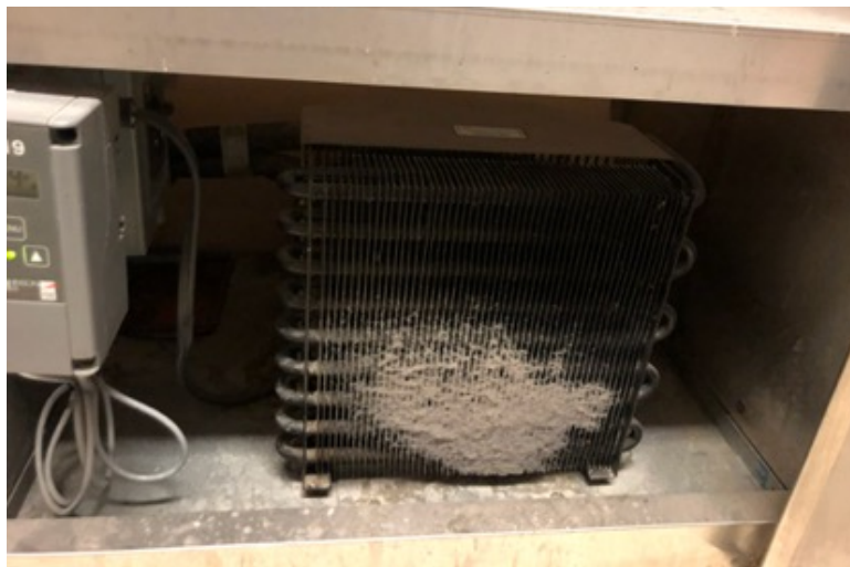
Photo 8: Exhaust under the clinic sink had accumulated dust (photographed June 8, 2021)
