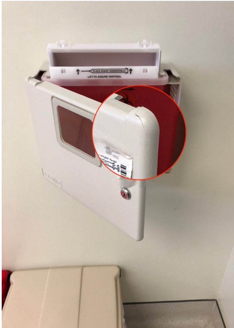
Photo 12. Damaged biohazardous sharps wall mount (photographed on March 4, 2021).
