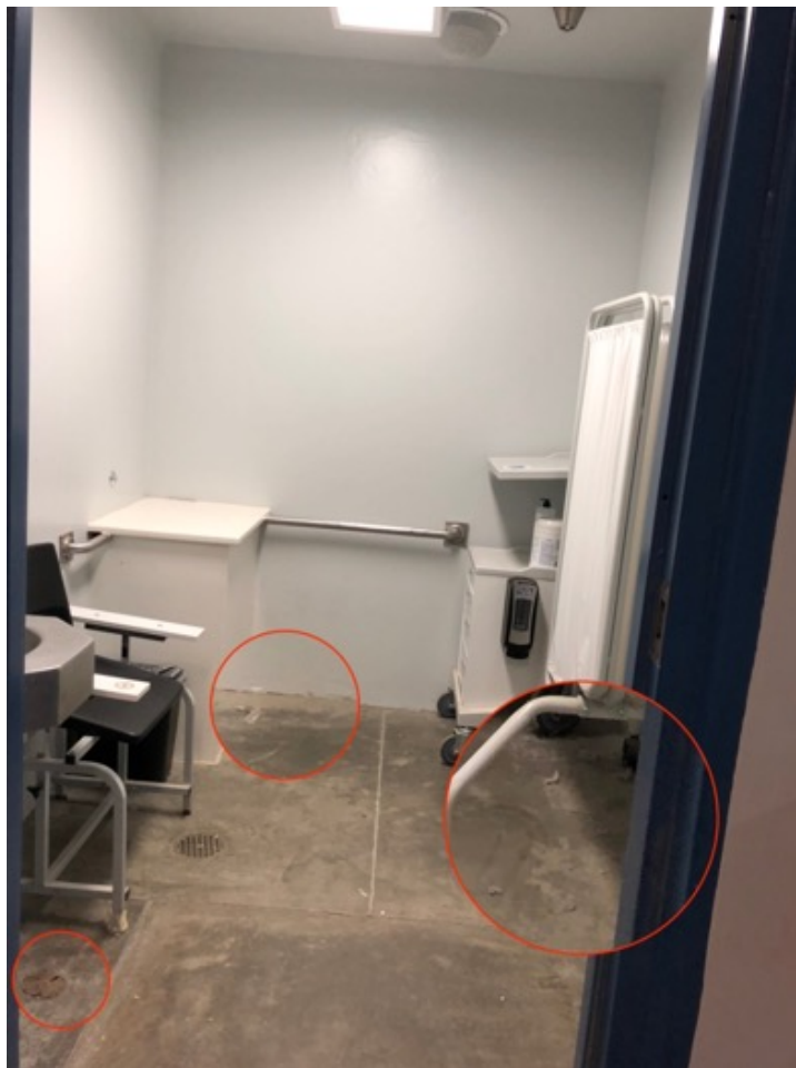
Photo 13. Treatment room was not free of grime and dust build-up (photographed on March 3, 2021).
