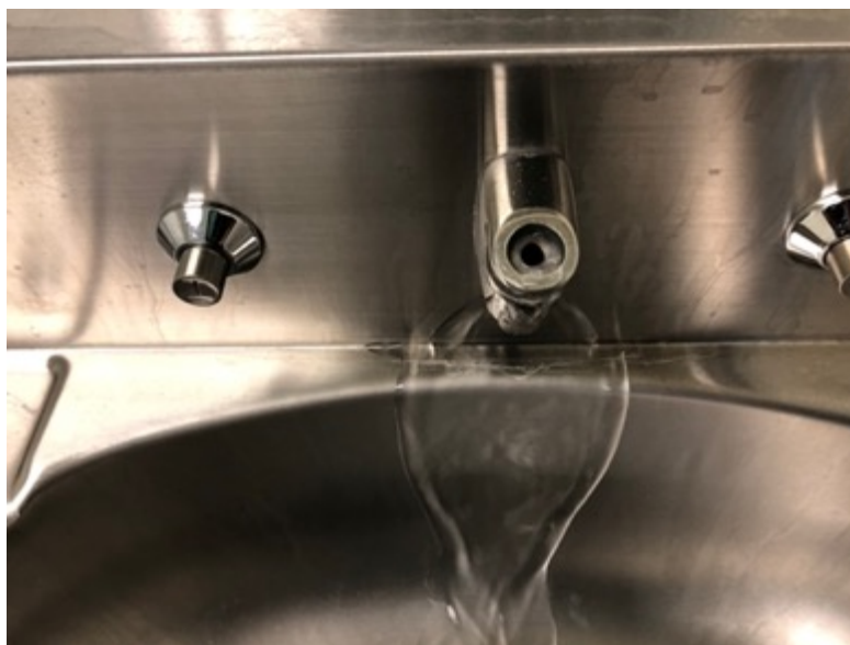
Photo 13. Nonfunctional patient restroom sink with water leaking from the bottom of the spout (Photographed May 11, 2021).
