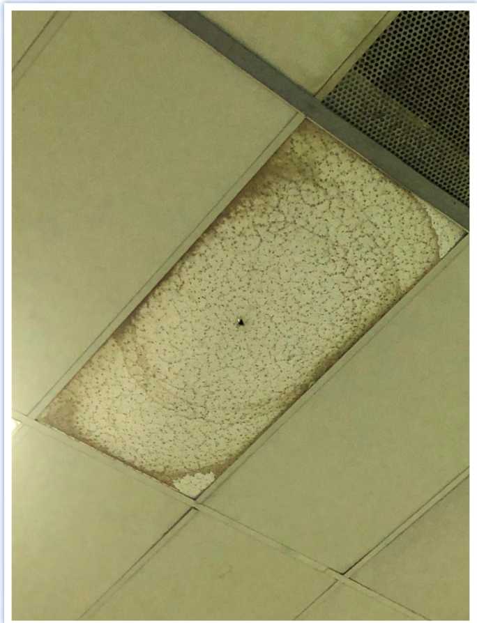
Photo 10. Medical warehouse reported water damage to the ceiling (photographed on October 14, 2020).
