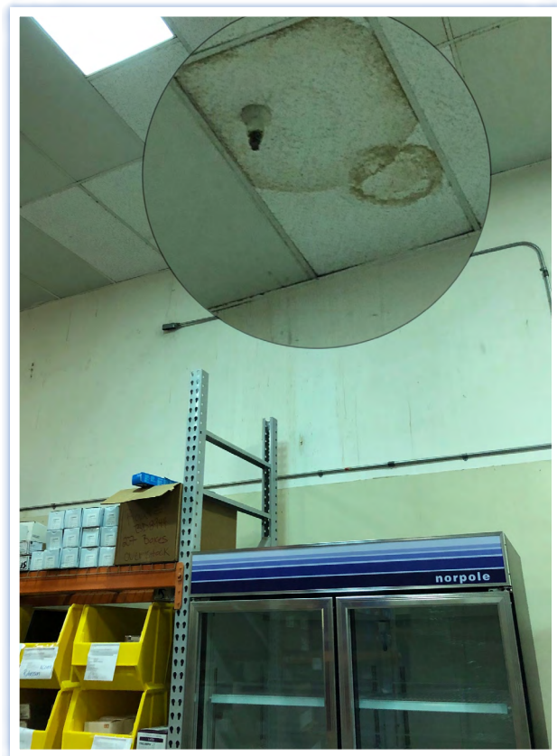
Photo 11. Medical warehouse reported water damage to the ceiling (photographed on October 14, 2020).
