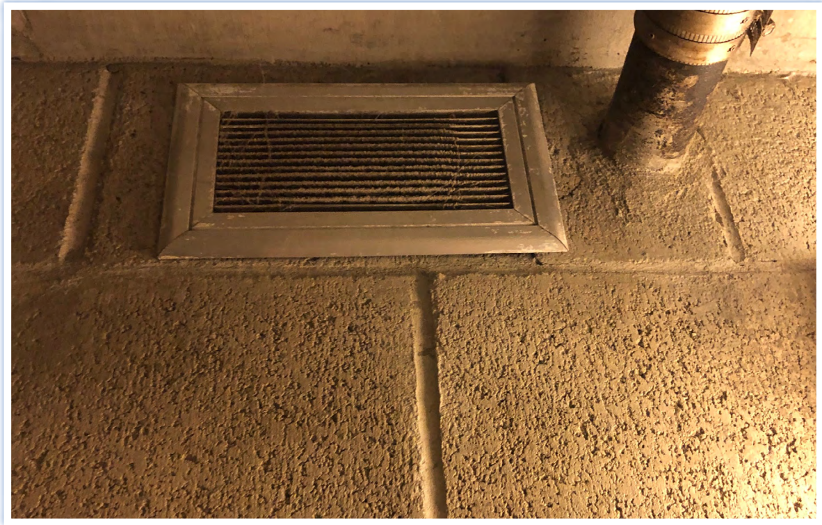
Photo 12. Staff restroom vents had accumulated dirt (photographed on October 16, 2020).
