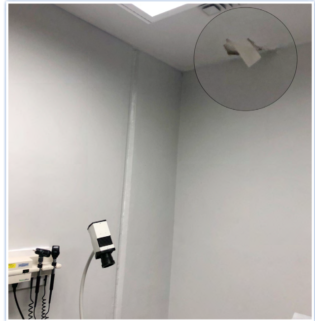
Photo 4. Residual water damage (photographed on September 17, 2020).
