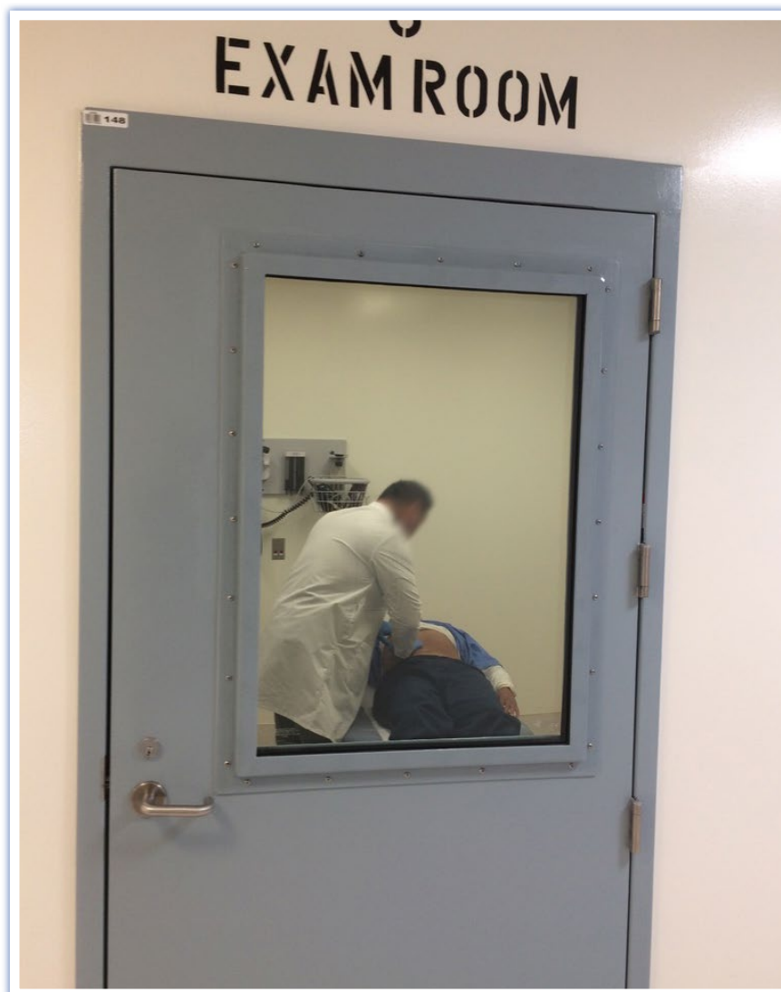
Photo 3. Examination room lacking visual privacy (photographed on September 10, 2019).
