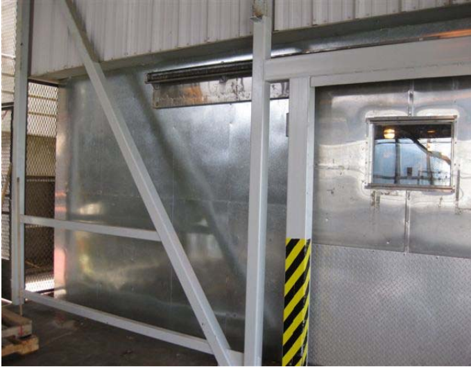
Figure 2 – Temporary Repairs on a Refrigerator
