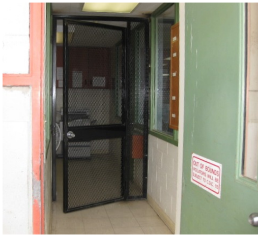
Figure 2 – Metal Grate in Program Office. Photo: OIG October 2010
