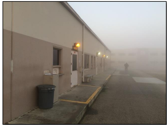
Figure 2: Insufficient overhang to protect patients waiting at pill lines from inclement weather or extreme heat
