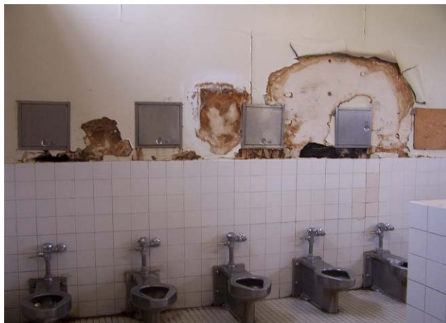
Bathroom in Pine Hall dorm showing water damage from plumbing leaks
