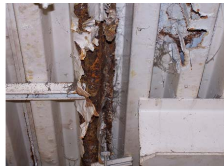
Rusted subflooring, South Dorm
