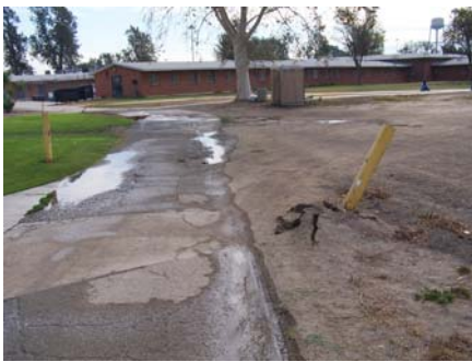
Example of cracked, rutted, and uneven roadway.
