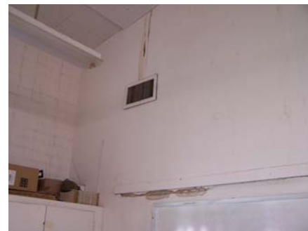
Water damage in education room caused by leaking roof.
