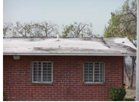
Housing unit roof that needs repair.
