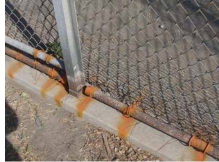
Rusted wire on perimeter fence.
