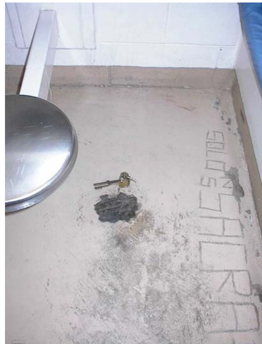
A hole in the floor of the Sacramento living unit after it was patched by plant operations.
