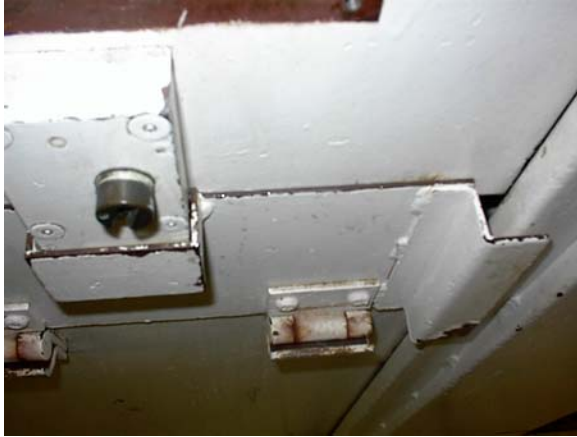
A door in the Kern living unit showing gaps next to the food tray slot that provides an opportunity for gassing assaults.
