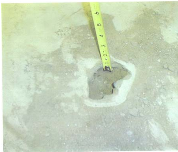
Picture provided by California Youth Authority staff illustrating a hole dug by a ward in the floor of a room in the Sacramento living unit. This hole had been repaired prior to the initiation of the audit.
