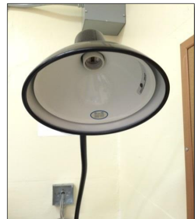
Figure 1: Exam Room light fixture without a light bulb
